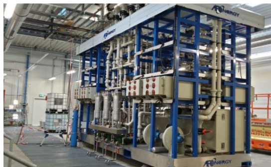
Fig. 44 AFC Energy's "POWER-UP", the world's largest operational AFC system at Air Products' industrial gas plant in Germany (1).
